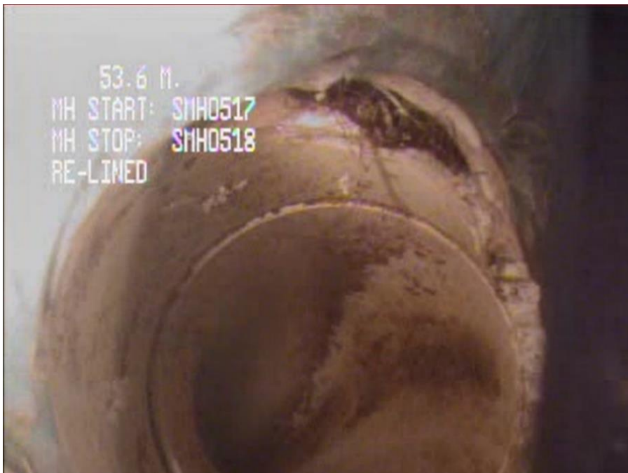
Figure 6-5: Overcut Lateral Connection with Damage to the Lateral and Root Intrusion
