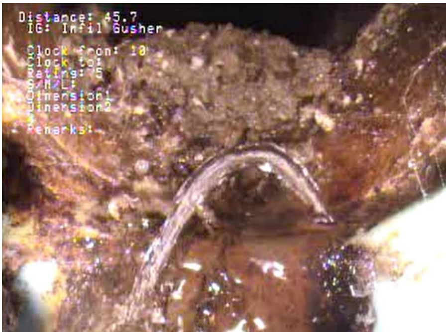
Figure 6-7: I&I at a Lateral Cutout (Picture 2)
