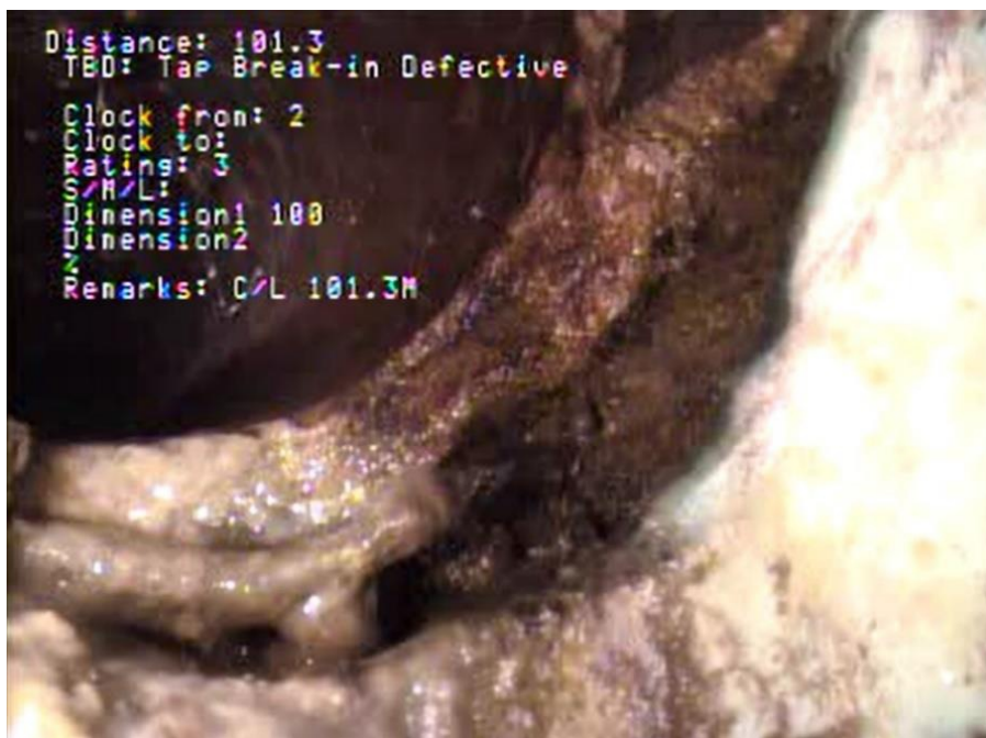
Figure 6-9: Soil Visible at a Lateral Interface – No Structural Connection of Lateral and Main
