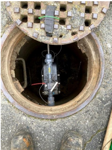
Figure 7-2: Echo Level Logger Setup
