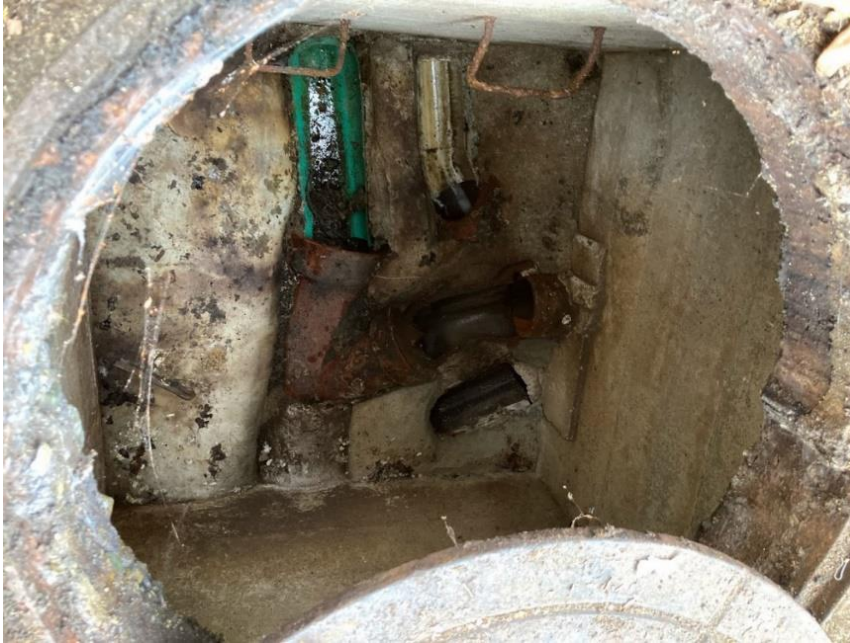
Figure 5-3: Combined Manhole at 861 Kindersley Road
