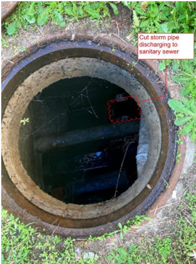
Figure 5-2: Combined Manhole at Archie Browning Sport Centre
