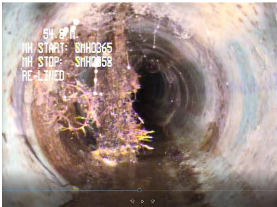
Figure 6-8: Root Intrusion at a Lateral Interface – No Structural Connection of Lateral and Main
