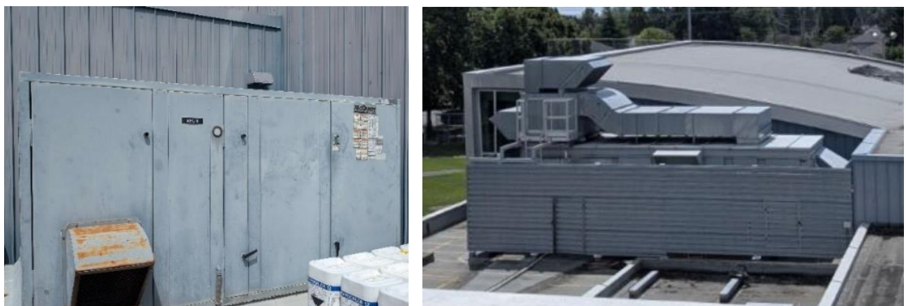
Figure 3-2 AHU-03 and HRV on AHU-1
