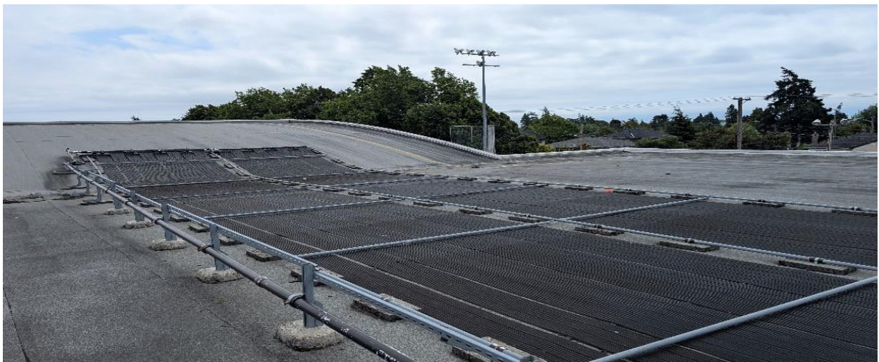
Figure 3-12 Solar Water Heating Panels
