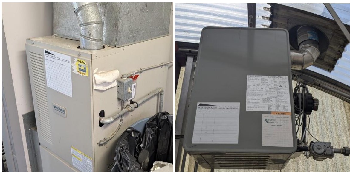
Figure 3-2 Office Area Furnace and Storage Room/Greenhouse Unit Heater
