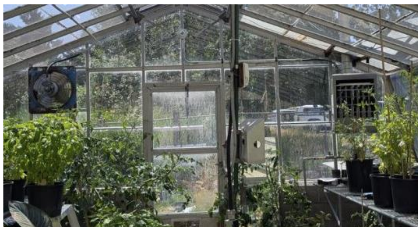
Figure 3-3 Greenhouse Exhaust Fan and Unit Heater
