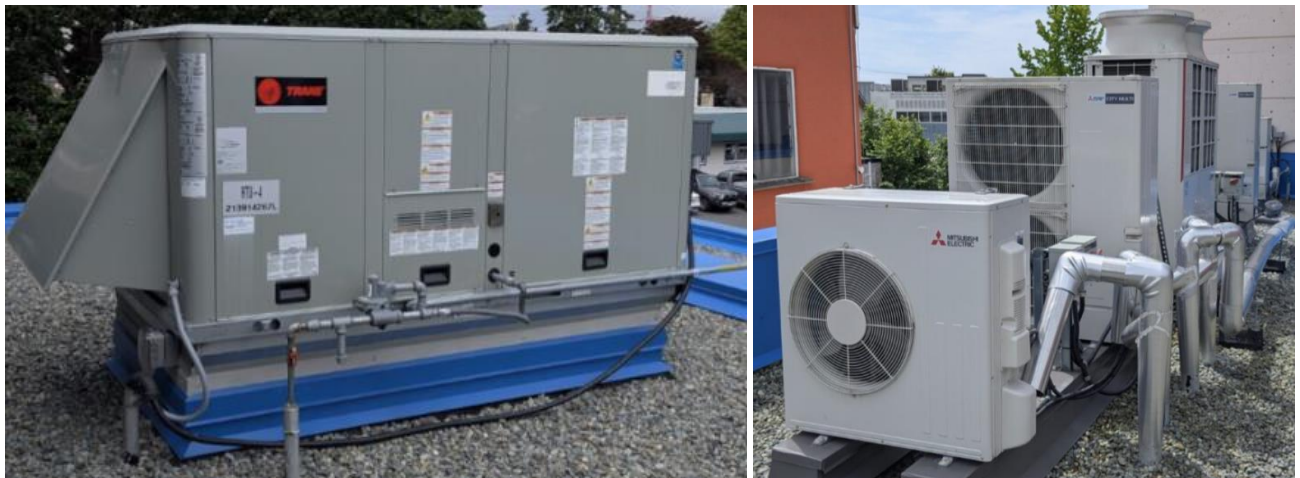
Figure 3-2 RTU-4 and Condensing Units
