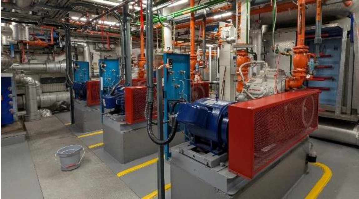
Figure 3-5 Ice Plant Archie Browning Sport Centre
