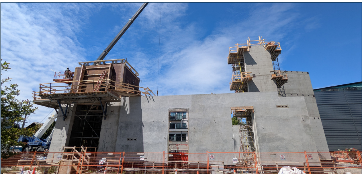
The Esquimalt Public Safety Building's construction made good progress in 2025. The building is slated to open winter 2026.
