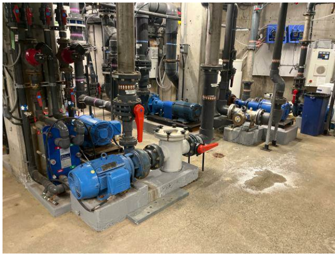
Photo #26: Pool Filter Room - Pumps
