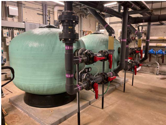
Photo #24: Pool Filter - Typical
