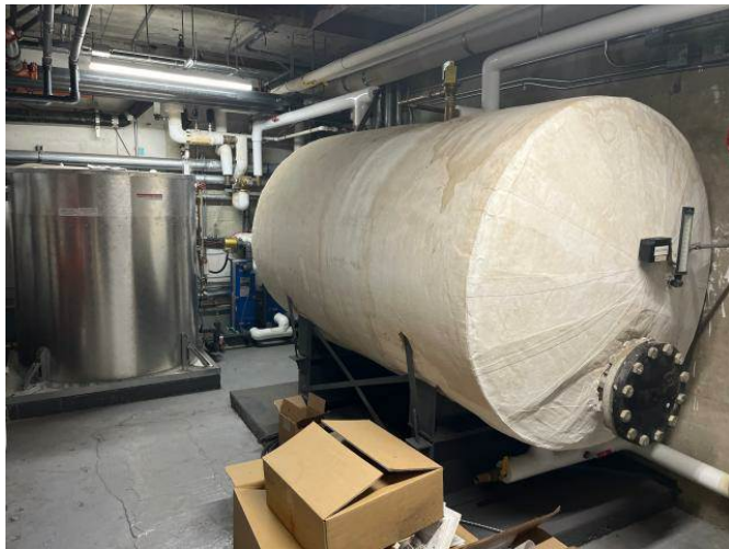
Photo #27: Domestic Water Storage Tank
