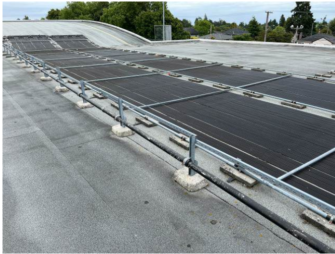
Photo #23: Solar Heat Recovery System
