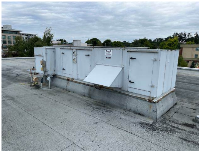
Photo #17: Roof-Top Air Handling Unit
