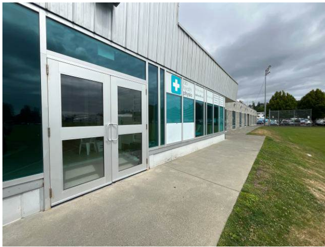
Photo #11: Aluminum Double Glazed Door - Typical
