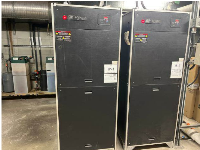
Photo #21: Heat Pumps HP1 and HP2 in Mech Penthouse
