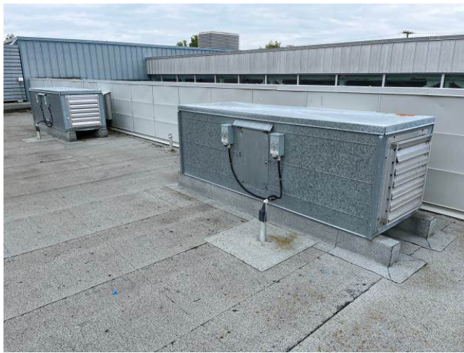
Photo #20: Pool Air Balancing Box
