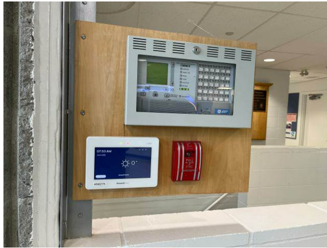
Photo #13: Fire Alarm Annunciator Panel
