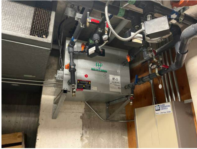
Photo #22: Heat Pump in Boiler Room
