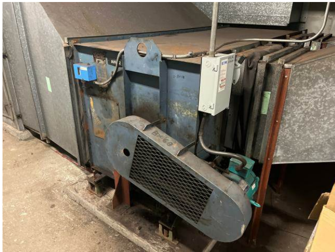
Photo #18: Indoor Air Handling Unit
