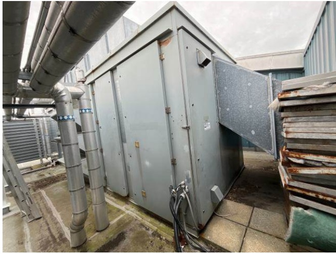
Photo #16: Pool Air Handling-Dehumidification Unit
