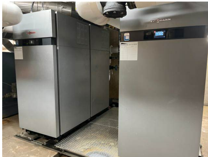
Photo #15: Central Heating Plant - Two New Boilers
