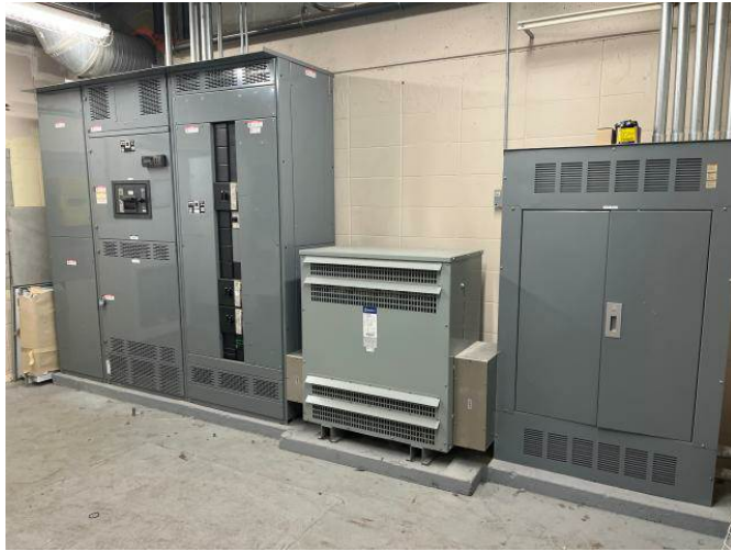
Photo #19: Main Electrical Room
