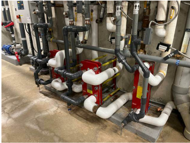
Photo #25: Pool Filter Room - Heat Exchangers
