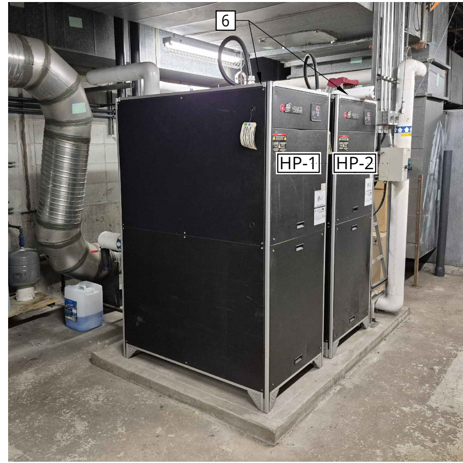
HEAT PUMPS HP-1 AND HP-2
