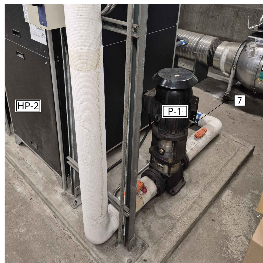
CHILLED WATER PUMP
