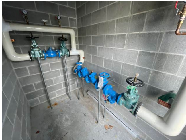
Photo #37: Incoming Water Service
