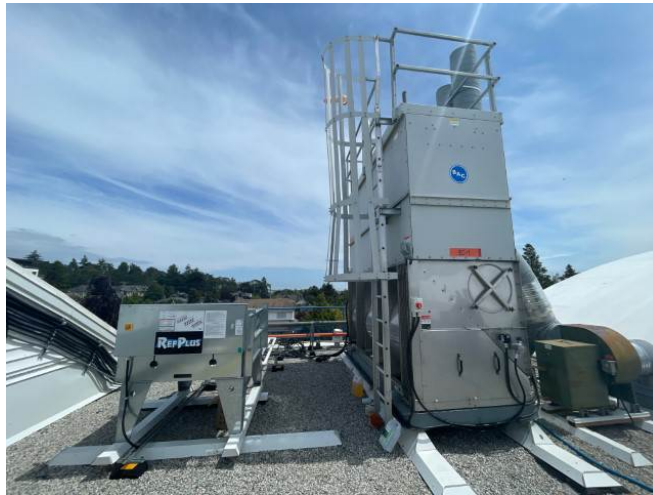
Photo #44: Ice Plant Condensor and Glycol Cooling Unit
