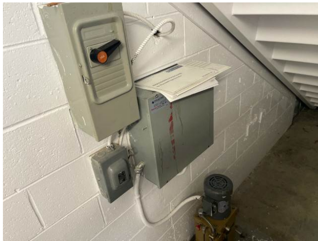
Photo #54: Elevator Machine
