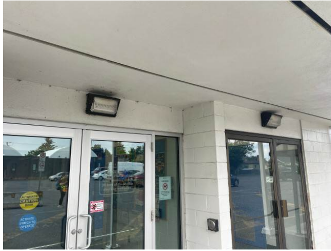
Photo #53: Exterior Lighting - Typical
