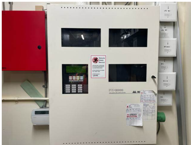
Photo #27: Fire Alarm Control Panel
