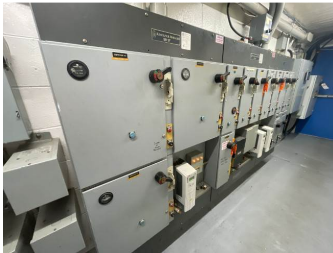
Photo #45: Ice Plant Controller Bank
