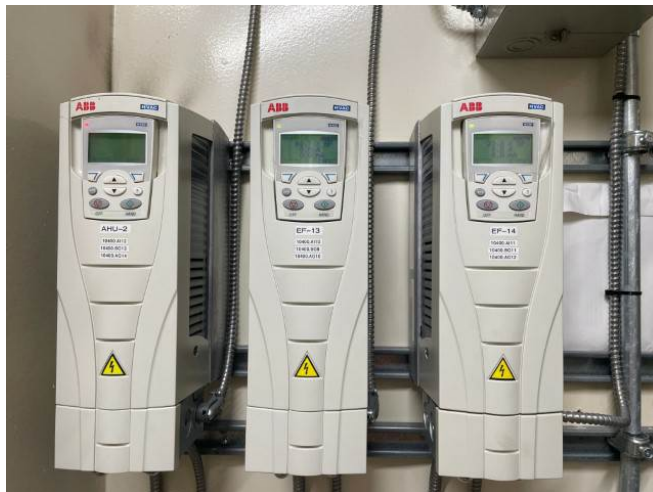
Photo #34: HVAC VFDs - Typical
