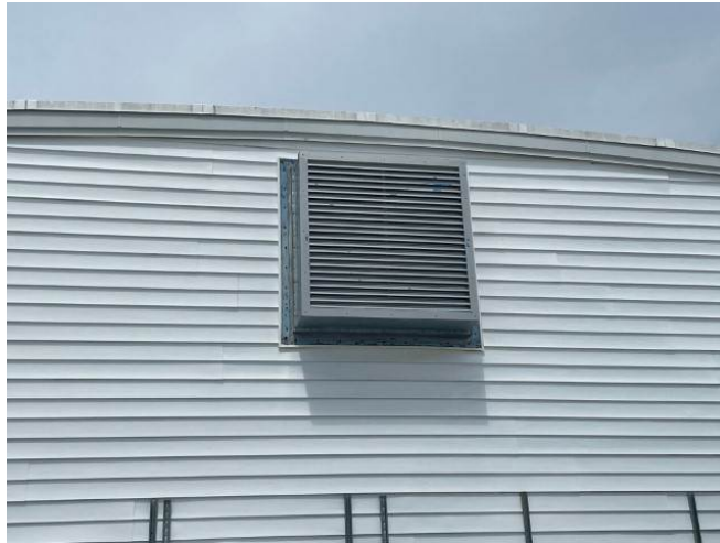
Photo #35: Rink Vent Louvre - Typical
