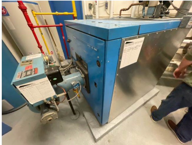
Photo #38: Gas-fired Boiler
