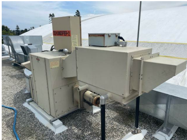
Photo #28: Curling Rink Dehumidifier Unit
