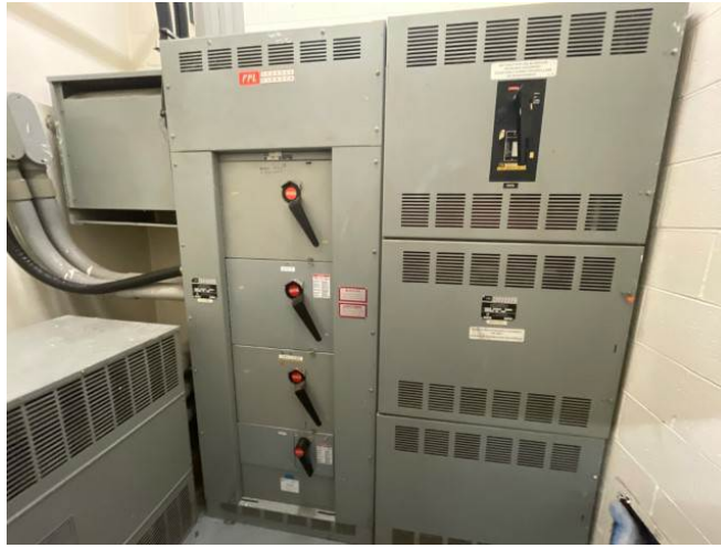
Photo #47: High-Voltage Switchgear and Transformer
