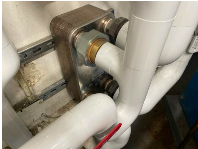
Photo #40: Hydronic Heating Heat Exchanger
