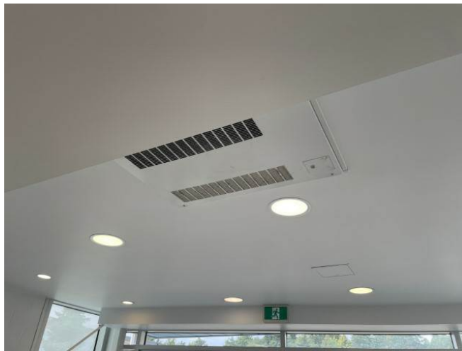
Photo #51: Interior LED Pot Lights - Typical
