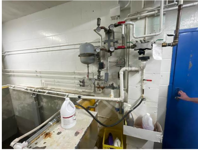
Photo #41: Ice Melt Pit
