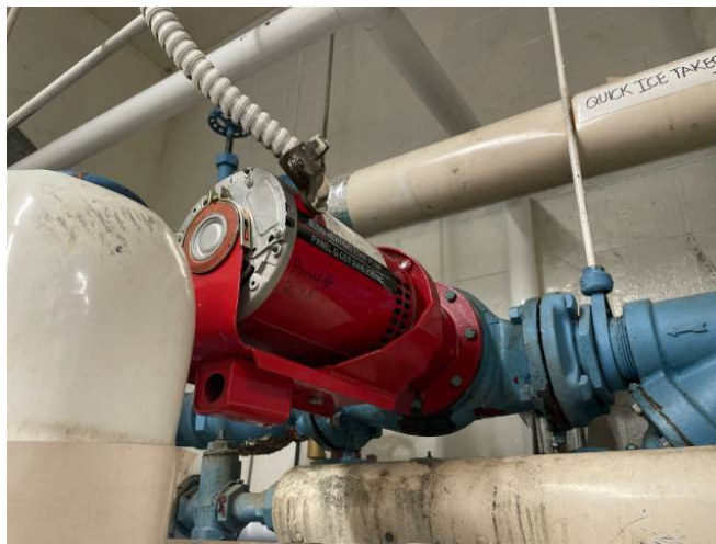
Photo #39: Hydronic Heating Circulation Pump - Typical
