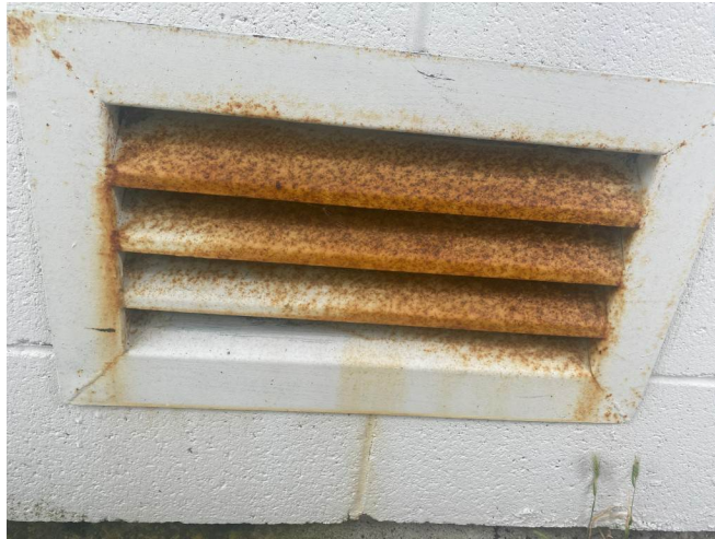
Photo #26: Ventilation Louvre in Poor Condition
