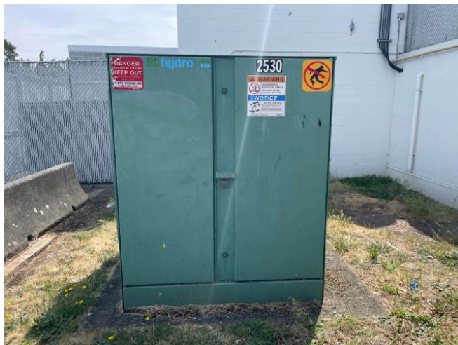
Photo #46: Site Transformer
