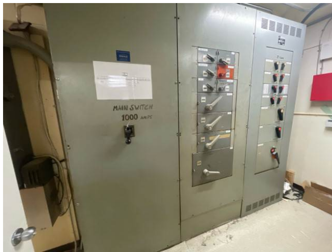
Photo #48: Main Electrical Switchgear
