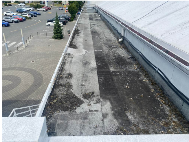
Photo #13: 2-Ply SBS Roofing in Poor Condition
