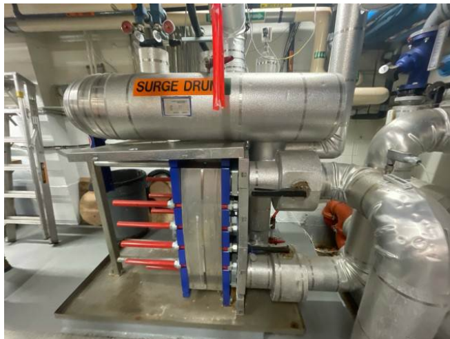
Photo #43: Ice Plant Evaporator Chiller - Typical
