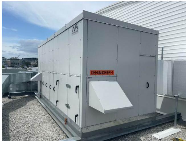
Photo #32: New Hockey Rink Dehumidifer Unit
