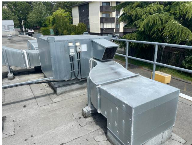
Photo #30: Rooftop HRV
