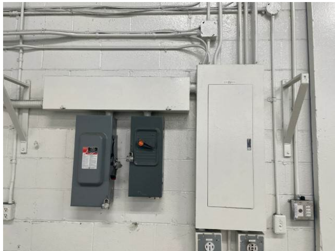
Photo #49: Electrical Distribution Panels and Disconnects - Typical
