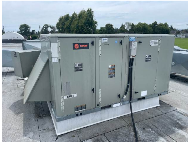
Photo #29: Packaged Rooftop Air Handling Unit - Typical
