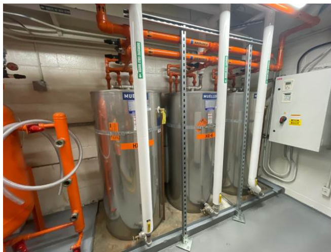
Photo #33: Ice Plant Heat Exchange Tanks
