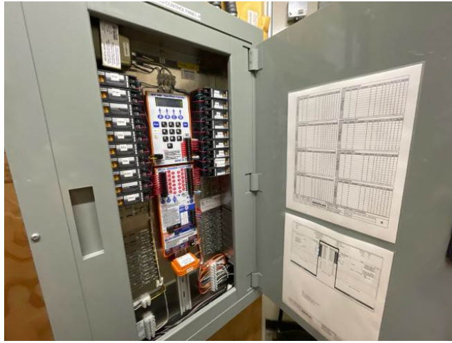
Photo #50: Lighting Panel - Typical
