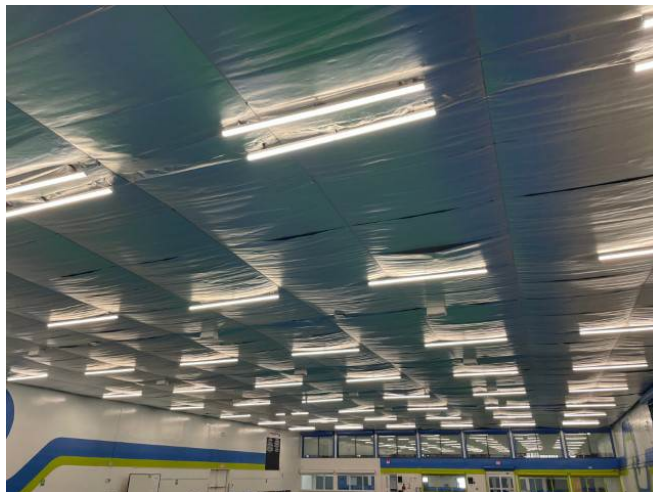
Photo #52: Interior LED Strip Lighting - Typical
