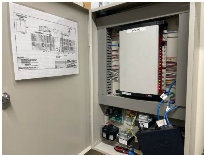
Photo #36: DDC Building Automation System Control Panel
