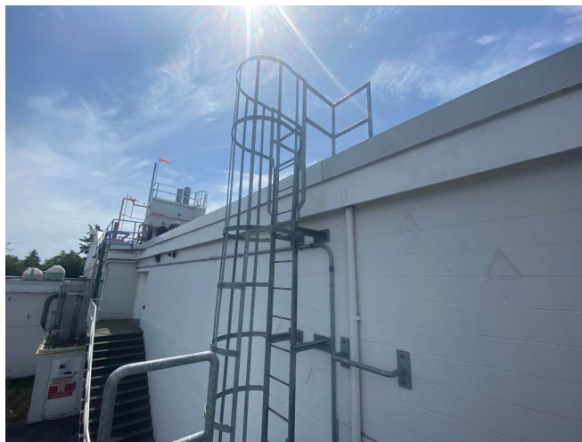
Photo #8: Caged Ladder
