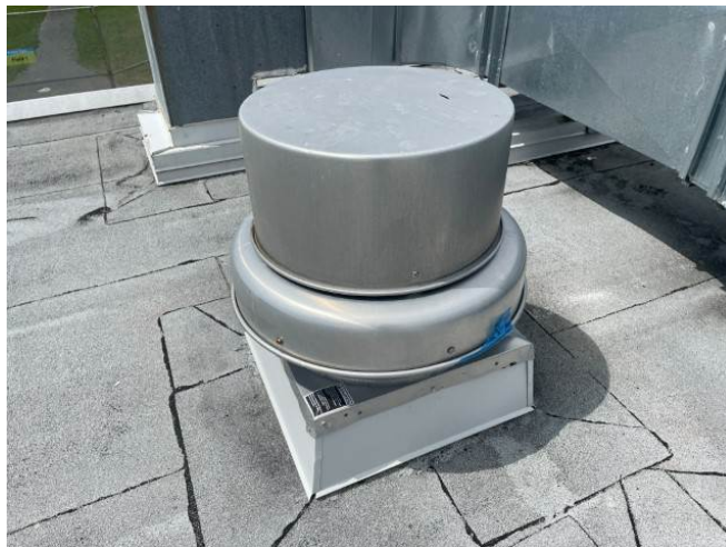
Photo #31: Rooftop Exhaust Fan - Typical
