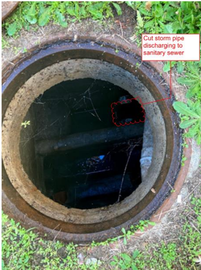
Figure 5-2: Combined Manhole at Archie Browning Sport Centre
