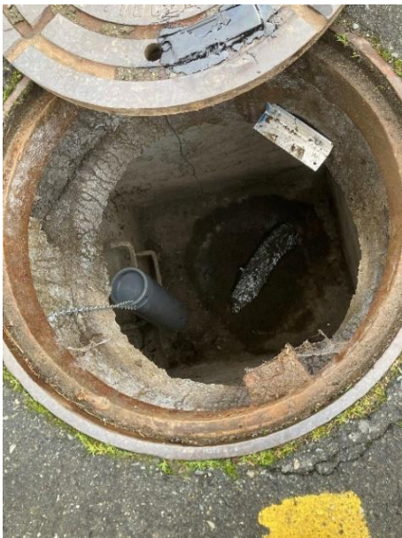
Figure 7-1: Ultrasonic Level Logger Setup
