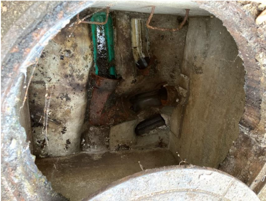
Figure 5-3: Combined Manhole at 861 Kindersley Road
