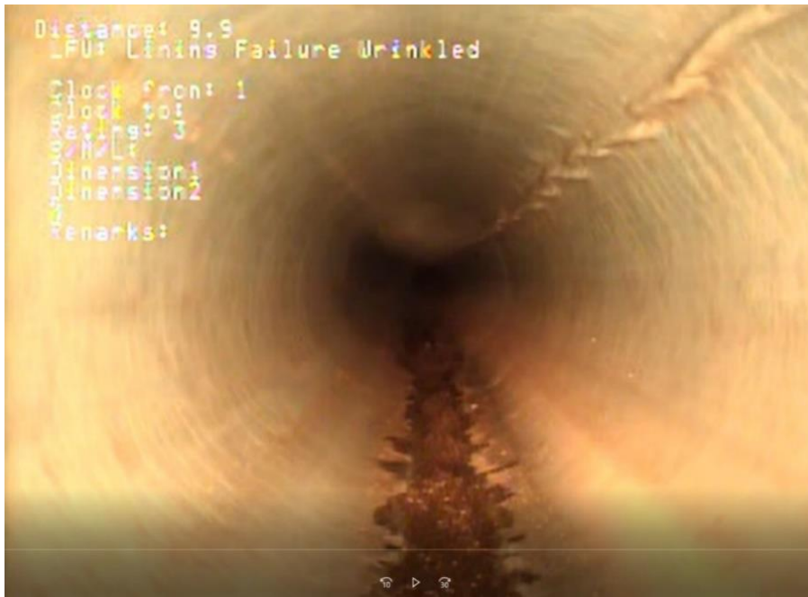
Figure 6-11: Liner Wrinkle – Not Affecting Structural Integrity or Hydraulics
