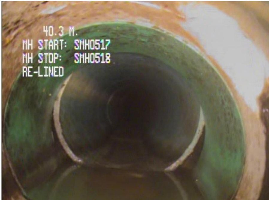
Figure 6-4: A New Wye Cut-in to a CIPP Lined Sewer that has Sagged (Picture 2)
