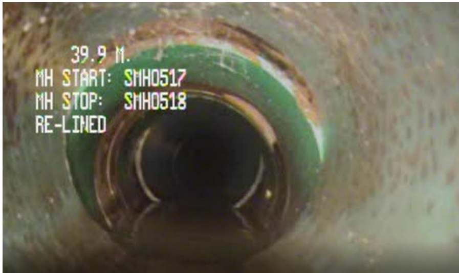
Figure 6-3: A New Wye Cut-in to a CIPP Lined Sewer that has Sagged (Picture 1)
