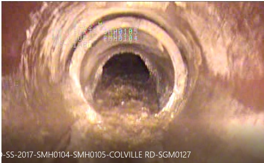
Figure 7-5: End of Line Colville Manhole SMH0104 – Full of Dirt
