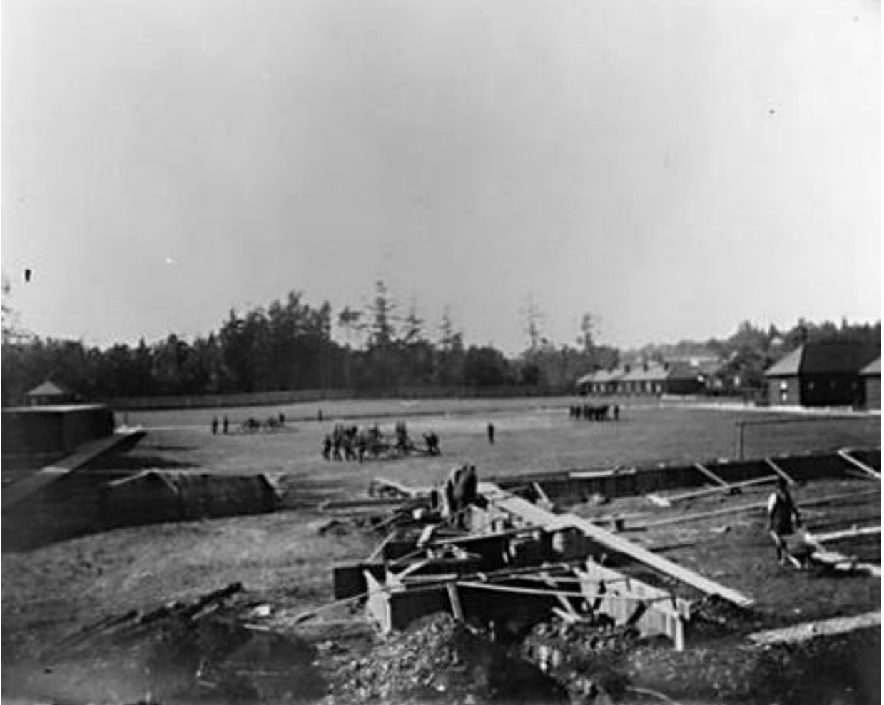
Work Point, looking west over the construction of the "Works Office" at Work Point Barracks circa 1893. In the background are the Royal Marine Artillery with their muzzle-loader carriage guns in the Parade Square and the Enlisted Men's Barracks to the far right. [Young Collection, Esquimalt Archives 994.4.7]
